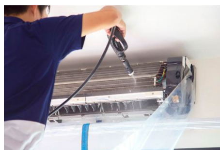
Regular servicing boosts AC performance.
