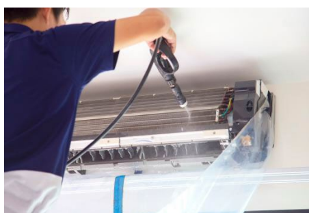
Regular servicing boosts AC performance.
